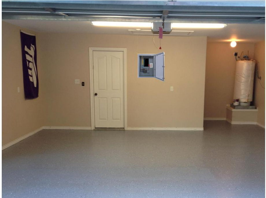
5G box in the garage
