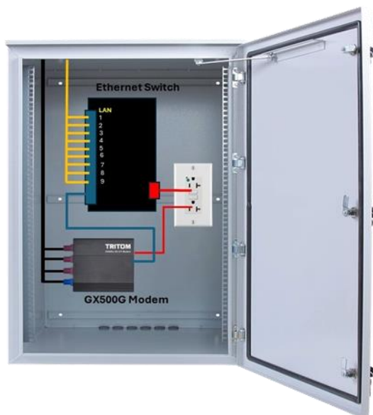
5G modem and network switch box
